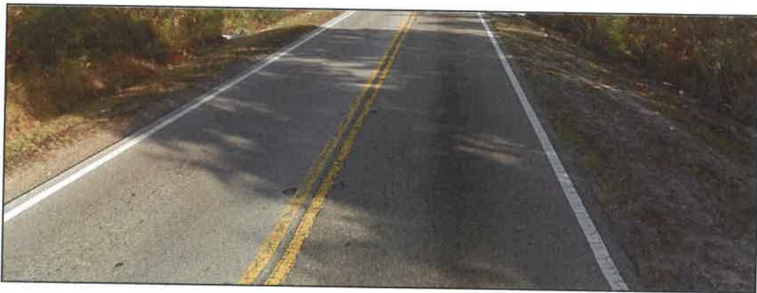
Figure 4- 1: Pavement Condition of Orange Avenue
